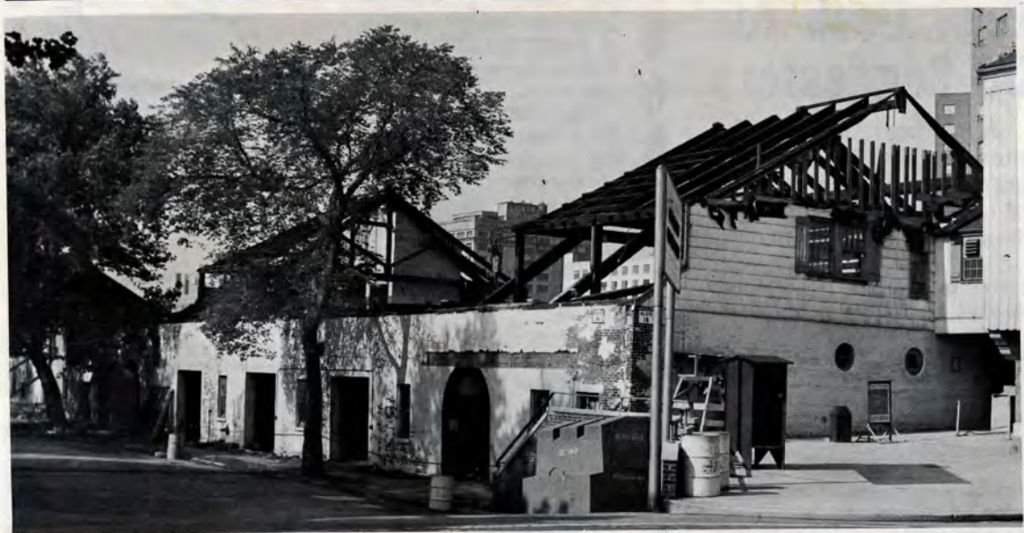
RAZING THE ROOF. After all these years, 130 to be exact, Building 16 located at the Sands Street gate, is departing from the Shipyard scene, being torn down as progress takes its toll. This is what was left of the building last Friday. What will go up on the site hasn't as yet been determined. Razing of Building 16, which was built in 1833, leaves Building 15 at north side of Sands Street gate as oldest employee-occupied building in yard. Building 15, which houses Employee Services Division and Board of Civil Service Examiners was also built in 1833 and like its neighbor was originally a timber shed. Now instead of 2 x 4's, the building has a lot of 5 x 5's.
